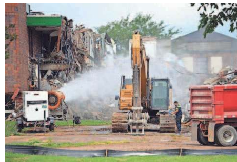
In June 2019, crews demolished the last of the buildings used by the State Home now on the property of Lakeland corrections facility.
